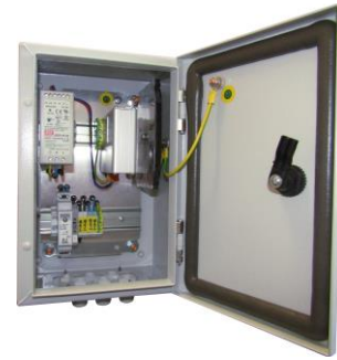
Mounting in Outdoor Switchgear OH3215
