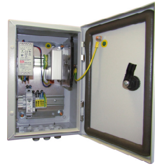
Mounting in Outdoor Switchgear OH3215
