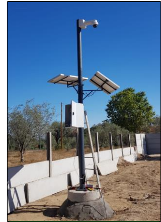
OFF-GRID System in Portugal
