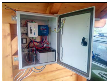
LoRaWAN System in Malá Skalice
