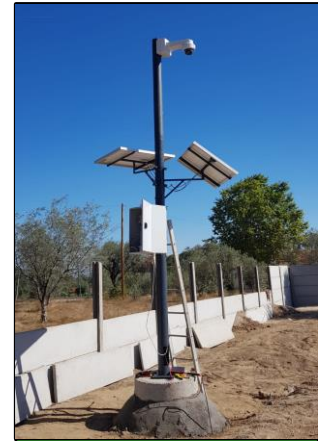
OFF-GRID System in Portugal
